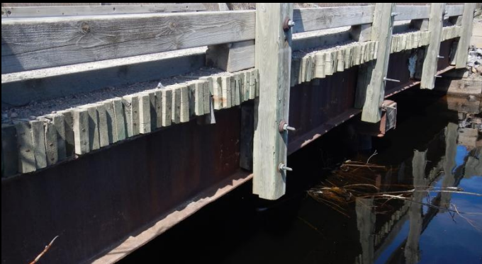
Photo 3: Downstream face of existing 9.6m span stringer bridge. Centre pile cap visible at midpoint of span. Stringer bending/distortion is also visible.
