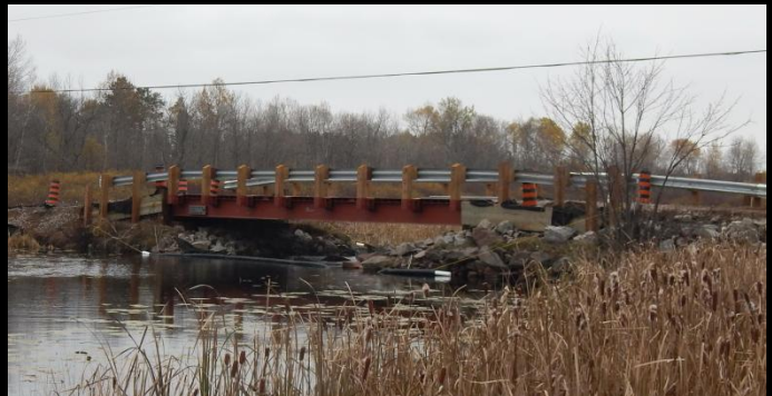
Photo 2: Upstream face of new 15.2m span Lessard Modular bridge looking North-easterly. Additional clearance below bridge visible.
