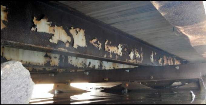
Photo 5: Photo showing centre pile cap and batter piles under mid span of existing bridge. Note poor condition of bridge stringers and limited clearance.
