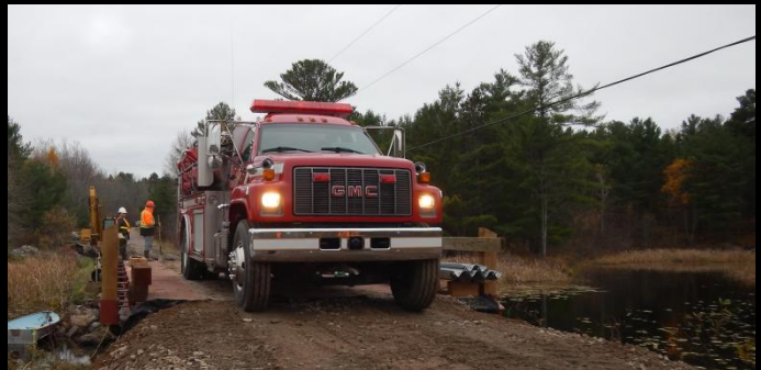
Photo 8: Municipal fire truck (Full of water) leaves its temporary post on the south side of the bridge (inaccessible during construction) while crew complete installation of new timber posts & steel guide rail.
