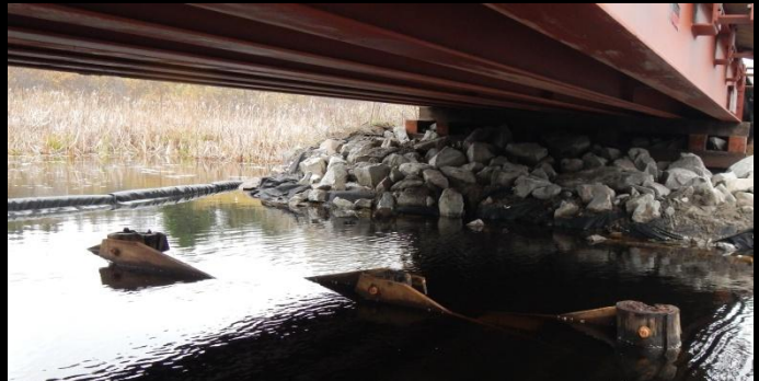
Photo 6: Photo showing the clearance under the new 15.2m span Lessard Modular bridge. Remnants of batter piles and new substructure are visible.
